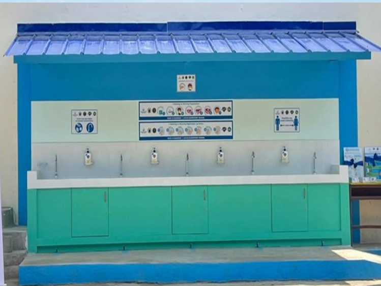
The handwashing facility's unique 'hybrid' design allows users to turn on the faucet by using a foot pedal.
